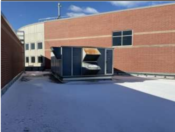
25 - ROOFTOP MECHANICAL EQUIPMENT
