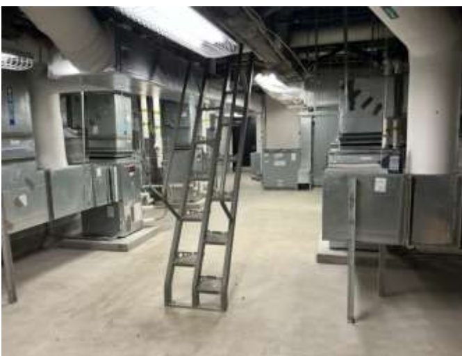
23 - SECONDARY MECHANICAL ROOM
