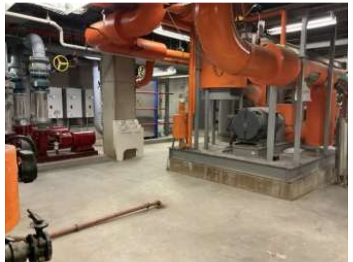
22 - MECHANICAL ROOM - PLUMBING
