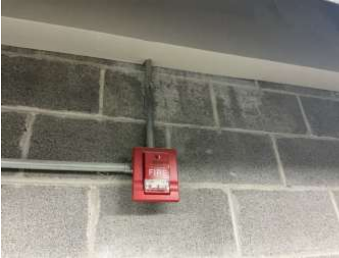
31 - FIRE ALARM DEVICES
