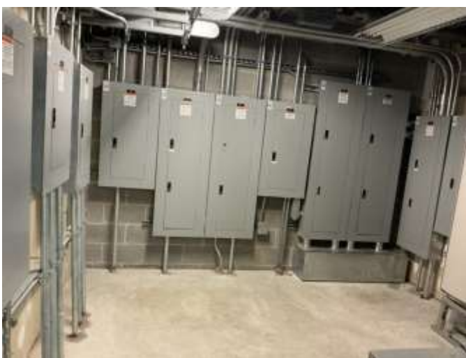
27 - SECONDARY ELECTRICAL ROOM
