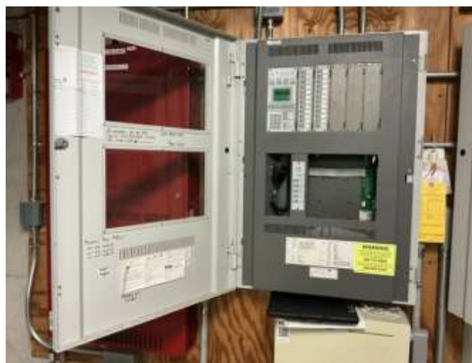
30 - FIRE ALARM PANEL
