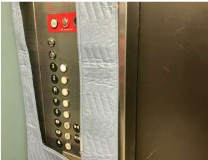
21 - ELEVATOR CAB PANEL
